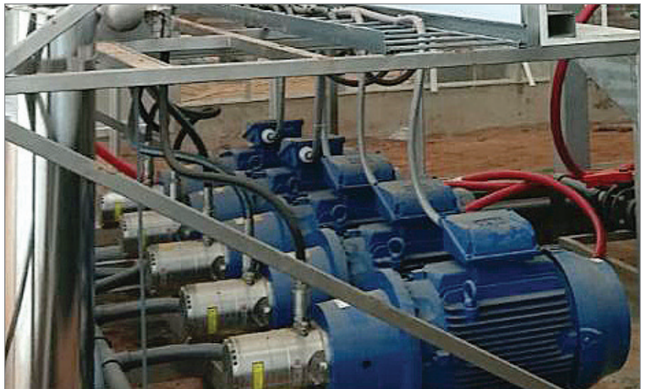
Five Danfoss PAHT 90 pumps help to provide pressure for the misting system.
